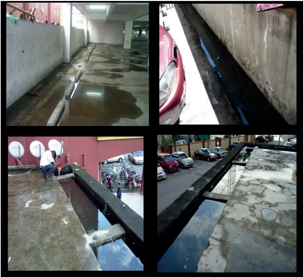
Figure 5. Stagnant water in the high-rise apartment buildings, which provides ideal habitats for Aedes mosquito breeding. Top: Apartment Building 1; Bottom: Apartment Building 2 (for location see Figure 3).
